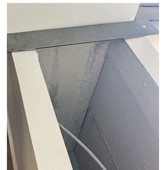
8 The 2 wall must be in level.
