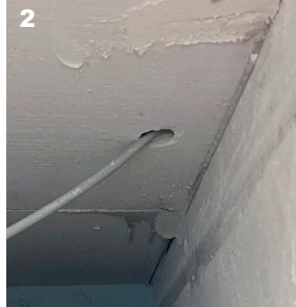
2 Too much space around the wiring, must be grouted.
