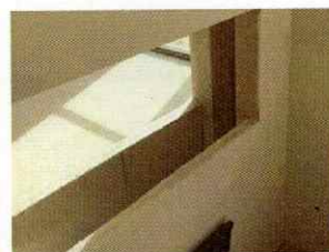
3. Side sections not sealed against false draft.
