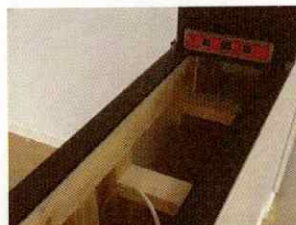
1. Combustible material inside recess (not permitted).
